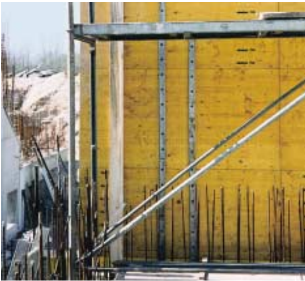
▲ The Coupler box is nailed to the formwork before reinforcement fixing commences.
